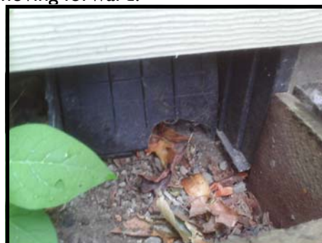
Photo of rodent entry on a bank-owned home.
