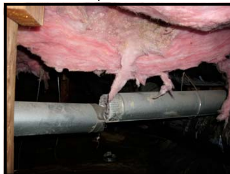
Photo of disconnect dryer duct in a bank-owned home.
