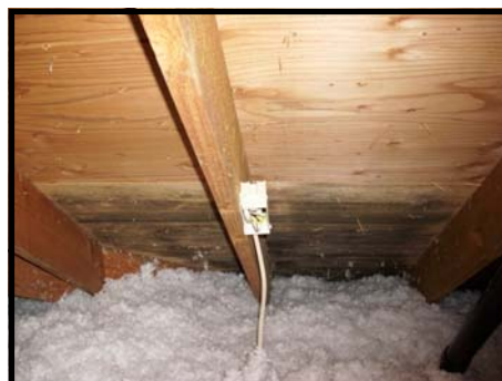
Photo of mold-like growth and uncovered electrical box in a bank-owned home.
